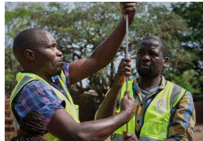
Repair of a faulty pump by two area mechanics in the Balaka district (Central region)
